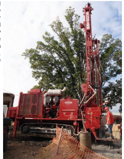
Allied Well Drilling’s new Schramm T450GT gets put through its paces at a geothermal installation just outside DC.
